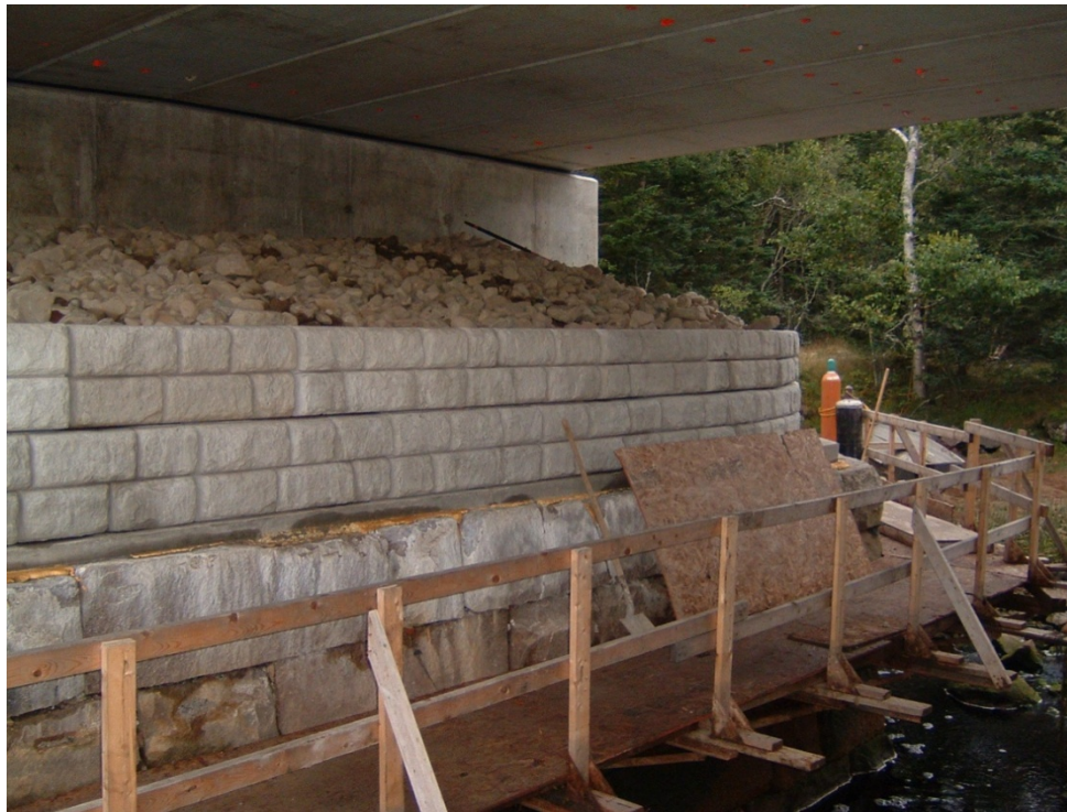
Figure 6. The Lamson Bridge Project maintained and preserved the existing cut stone block wall (on the bottom) for historic and environmental reasons.
