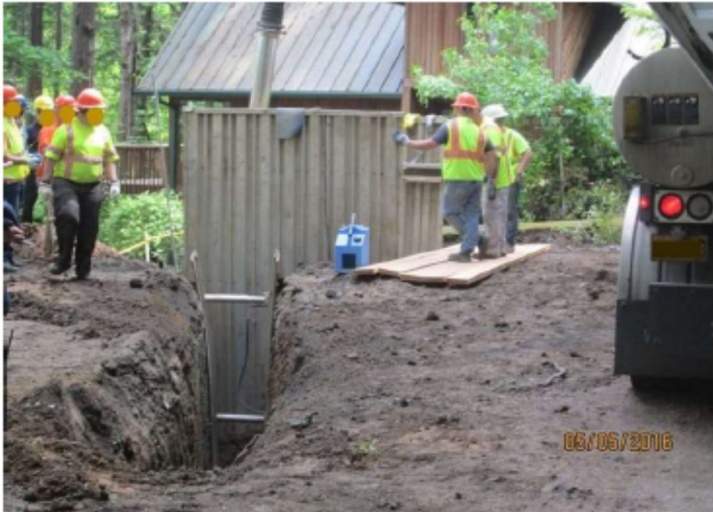
Figure 2. Emergency responders preparing to install a trench box before starting rescue and recovery work, to prevent risk of additional collapse and injuries
