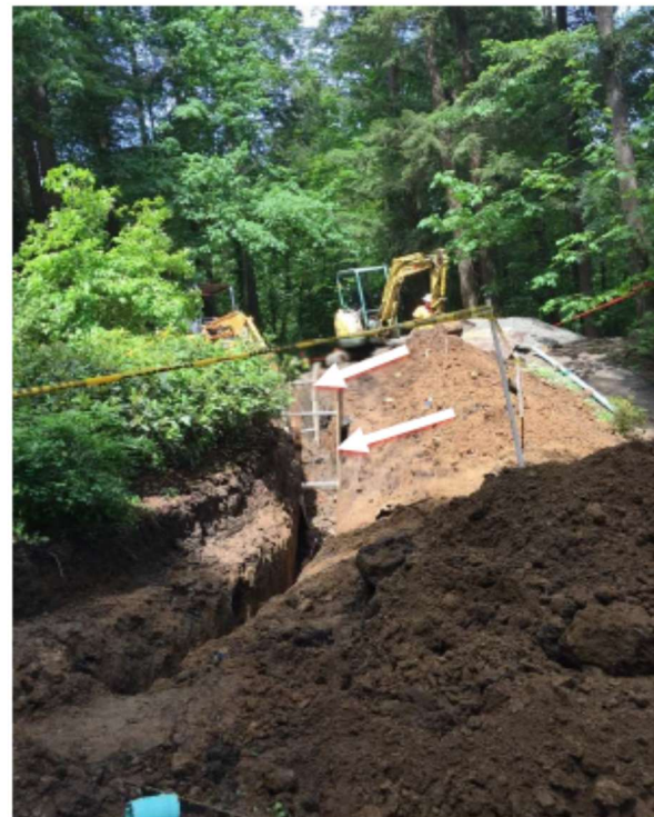
Figure 1. View from front of house: area of incident showing placement of shoring; collapse occurred in between the two pieces of shoring spaced 15 feet apart (indicated by arrows)
