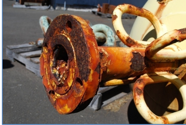
Figure 21: Corroded buoy mounting plate
