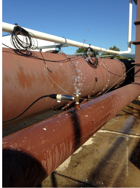
Figure A.4: Residual air accumulated at the crown of the horizontal pipe after each trial. Air was allowed to bleed through the valves installed along the horizontal pipe.
