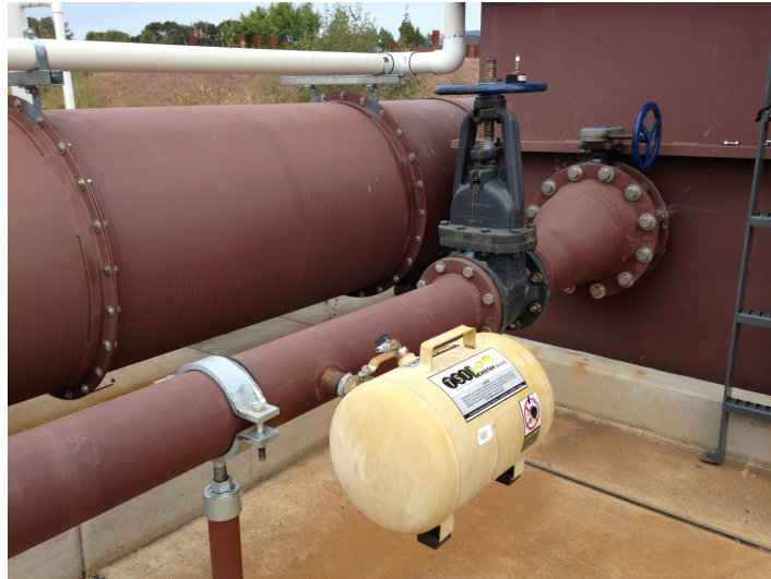
Figure A.1: The 12 inch butterfly valve, reducer, 6inch gate valve and air tank used in the physical experiment.
